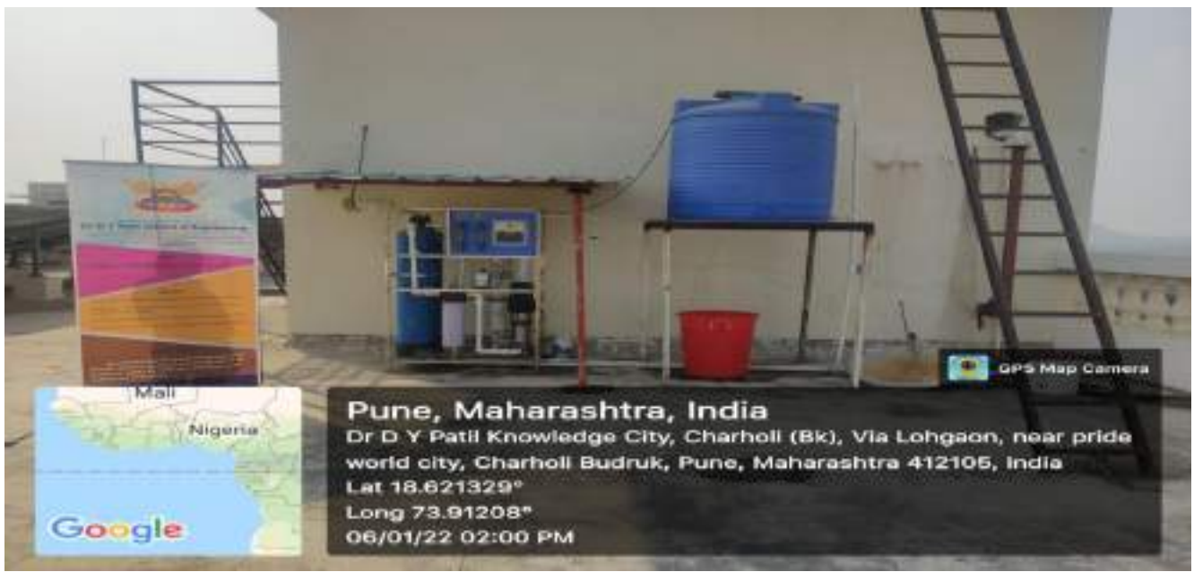
Watermark treatment plant on top of terrace
