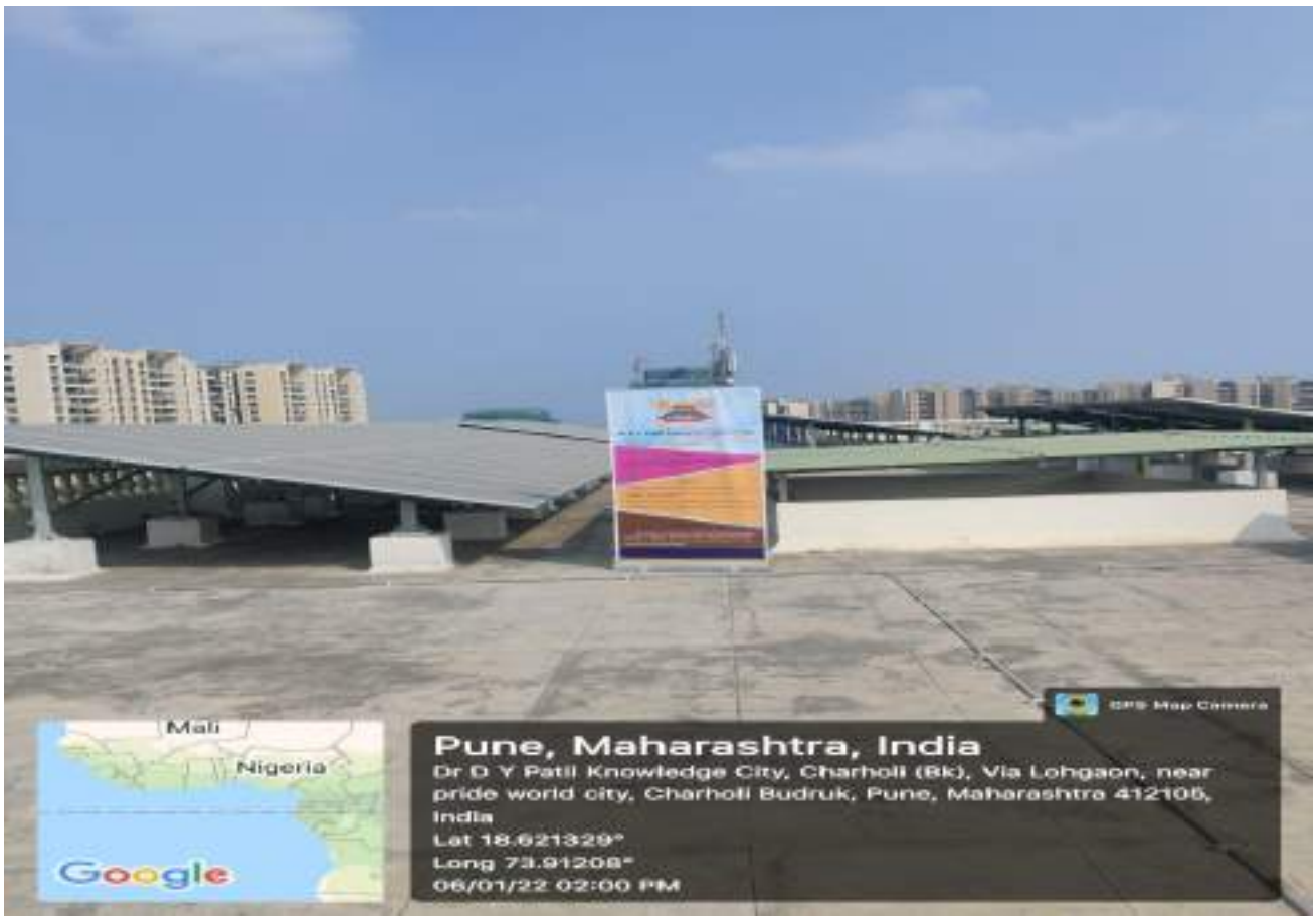
Solar System on top of Building
