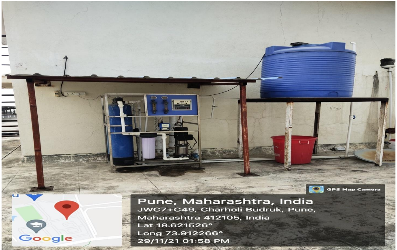
Overhead Water Tank Fitted with R.O. System
